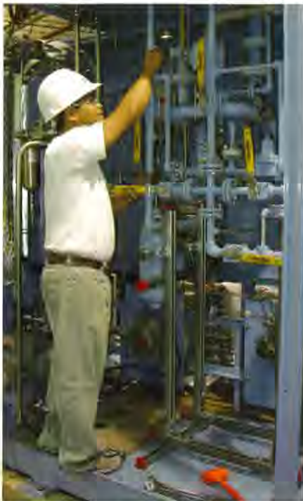
Specialist working on E/One Gas Station installation and start-up. The E/One Gas Station is a modular approach that combines monitoring and control systems into a single integrated platform, customized to meet specific site requirements and budget parameters. (Photo courtesy of Environment One Corporation.)
