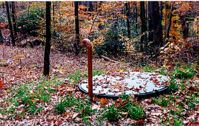
"All the E/One pump covers are at ground level," said Jeff Gaul, Director of Maintenance at Fallingwater. "They are even dark green which blends in to our environment."
