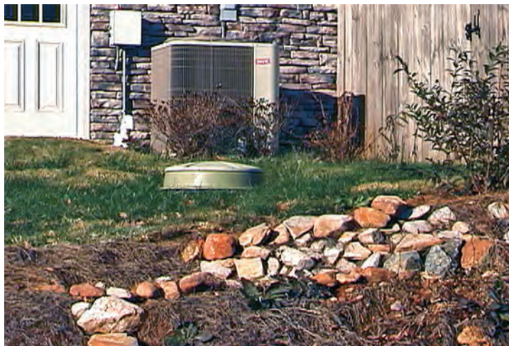
Image 1. A grinder pump station access lid
