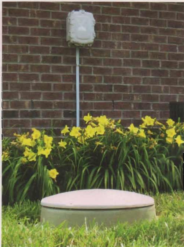
A grinder pump with an access lid for service is installed into the ground at each home.
