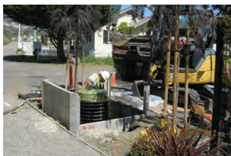
The heart of the ATS system is a tank about the size of a dishwasher that is buried in the ground, often within the same footprint as a decommissioned septic system. Photo: Stantec.
